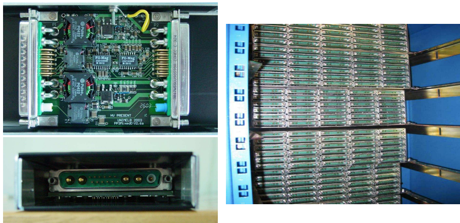
Figure 24. PP3 pictures. Top view with metal box open (top), the yellow wire connects the metal box to the cable shield. Front view of the PP3 (bottom), the two C-section pieces protect against magnetic fields. PP3 rack before cable installation (right).
